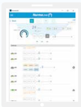
Control Tunable White.
